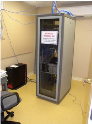
Secure and Climate-Controlled LAN Room – designed according to the current OCIO IT specifications.
